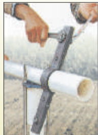
Always tight the metal clamp at marked place during lowering of pipe and lower the pipe by the help of chain pulley.
